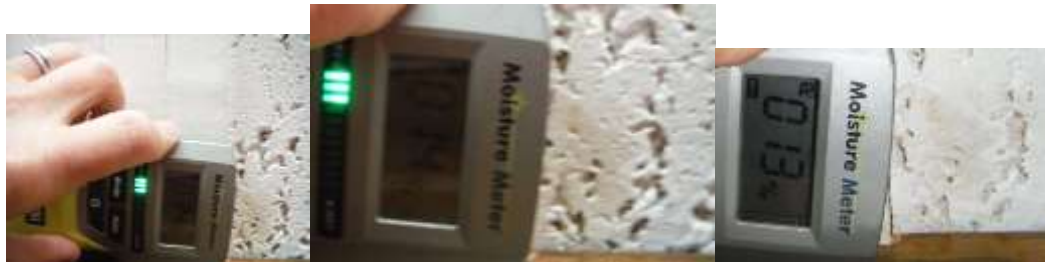
Figure 3 Active moisture on stains in kitchen.
