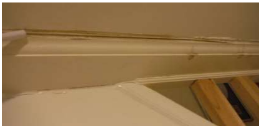
Figure 5 Moisture stains around ceiling/molding on stairwell to basement; tested dry at time of inspection. Ask history for stains; unknown.
