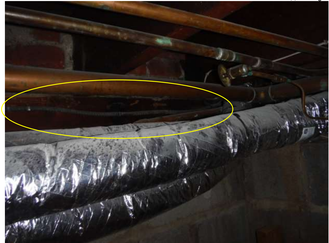
Figure 6 Termite tubes and sill damage in rear closet. Have extent of damage determined/repairs be structural carpenter. Rule out any concealed damage; inaccessible areas due to finished basement, shelving, storage. See separate NPMA-33 Termite report.
