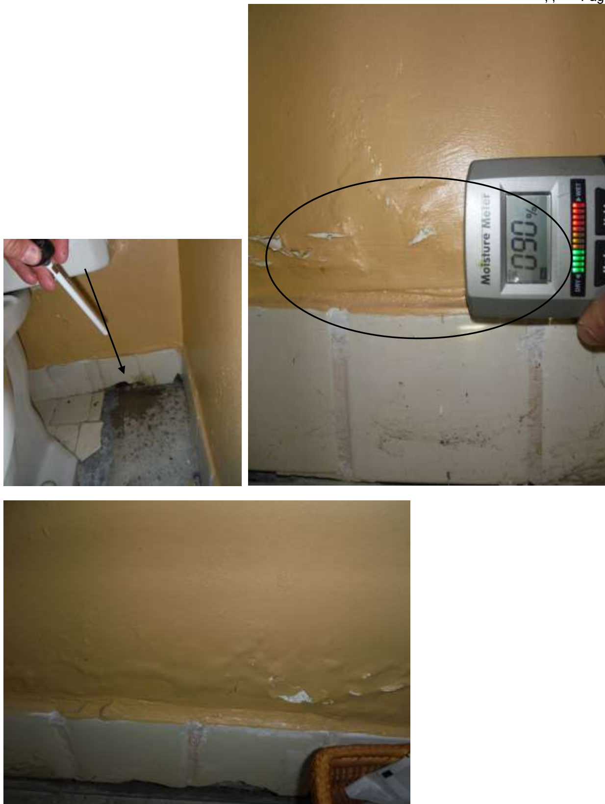
Figure 4 Water damage, efflorescence, peeled paint; seepage.
