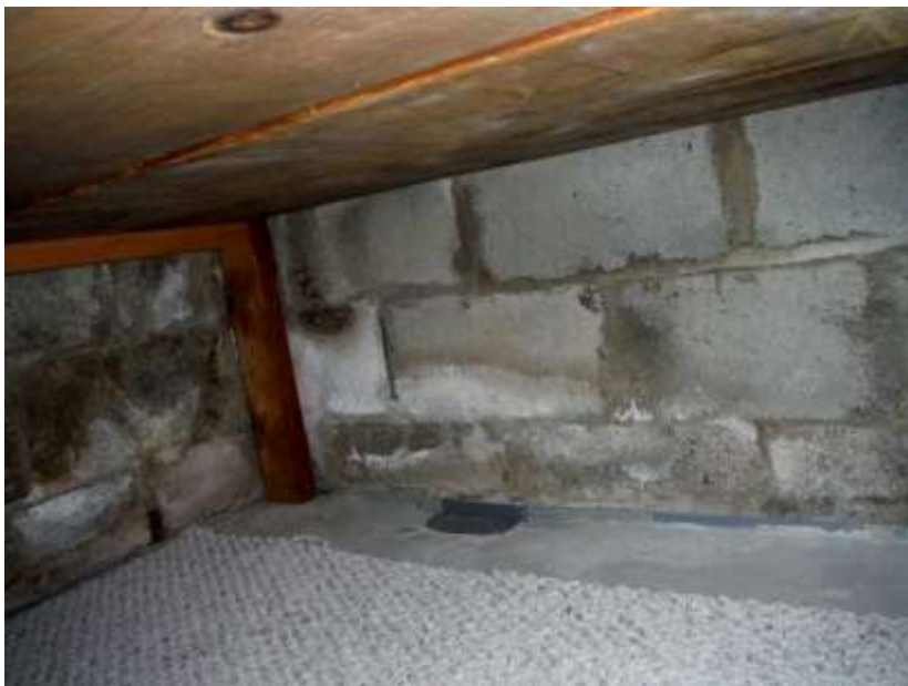
Figure 7 Example of seepage/water stains/efflorescence in basement; limited view due to finished basement.
