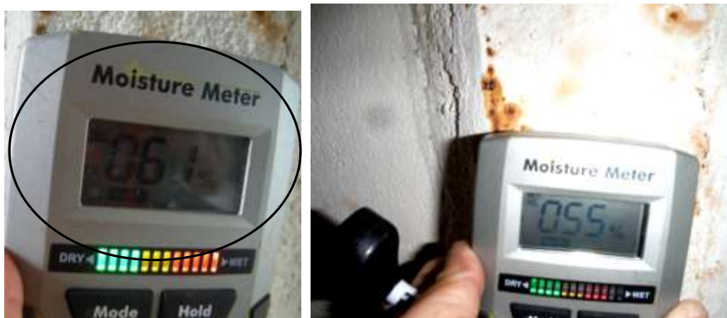
Figure 2 Rear butterfly roof leaking into garage and kitchen.
